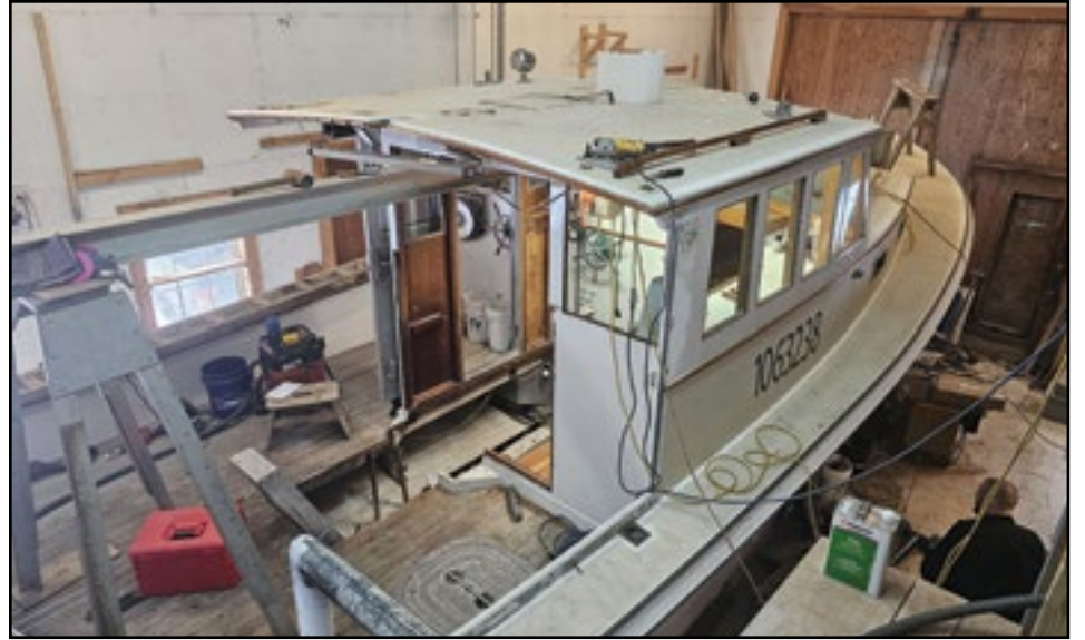
At John's Bay Boat Co. SARI ANN I is in for some major work. The engine, a 3208 Caterpillar was removed and workers have cleaned the engine room and making a major repair on the portside washboard.
