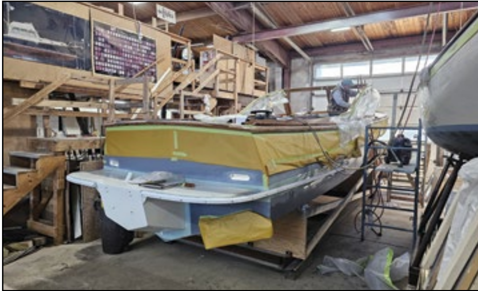
The 28-foot custom hull designed by Doug Zurn under construction at John Williams & Company in Hall's Quarry.
