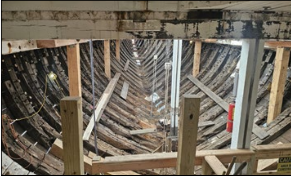
One of the big projects ongoing at the Henry Dupont Shipyard at Mystic Seaport is the rebuilding of the Gloucester schooner L. A. DUTTON. This is a view forward.
