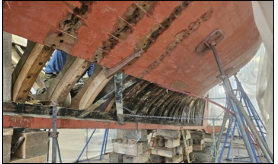
This is the schooner BRILLIANT, owned by Mystic Seaport in Mystic, Connecticut having work done at Rockport Marine in Rockport. This is a view showing how they opened her up to work on the frames.
