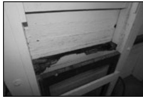
Area of cap-rail to be replaced. Typical example of rotten cap-rail/side decking to be replaced
