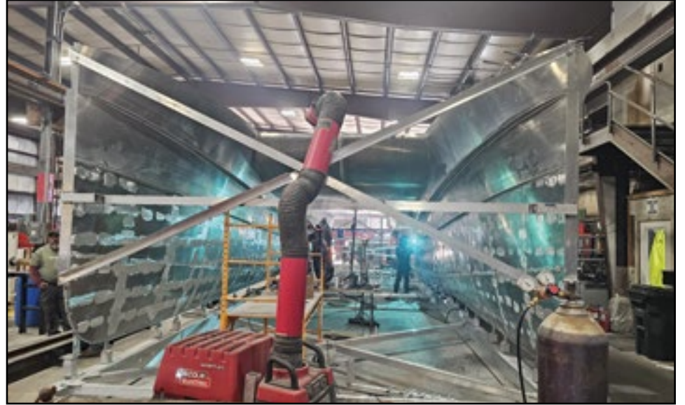
This is the 50-foot aluminum power catamaran under construction at Lyman-Morse Fabrication in Thomaston.
