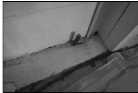
Typical example of rotten covering board to be replaced.
