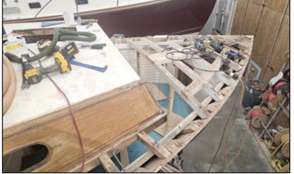
This is a bow view of the repairs made on the fore deck of the Bunker & Ellis power boat being restored at the Ellis Boat Company in Manset.
