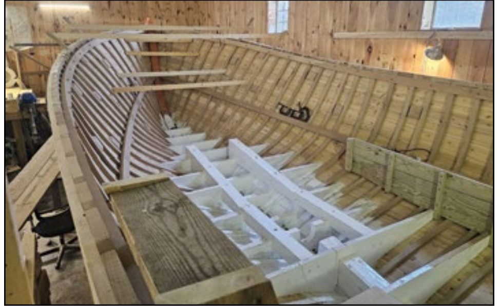
At Buxton Boat, they are progressing. The hull is done and they Peter Buxton and Tim Clark, are putting in the internal structure.
