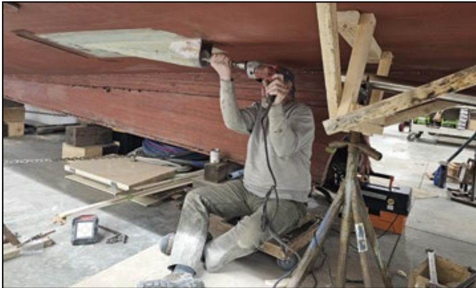
Richard Stanley working on the port shaft trying to align it with the starboard one. He has removed the cutlass bearing and is now sanding out the tube, before he starts putting her back together.
