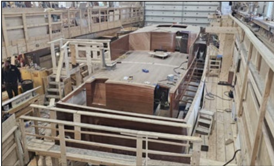
Over at Brooklin Boat Yard the Wheeler 55 motor yacht is progressing quickly. In my last post the house was sitting to her left under the balcony. The house has now been fitted to the hull as work continues on the interior.
