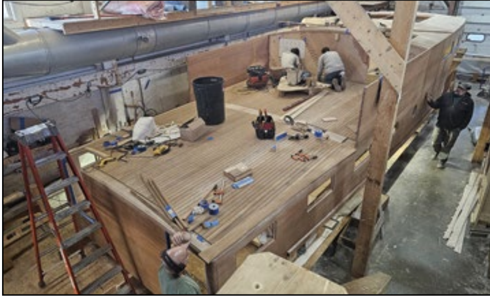
This is the cabin of the Wheeler 55 under construction at Brooklin Boat Yard in Brooklin. The plywood for this was cut by Hewes & Company in Blue Hill using their C&C machine.
