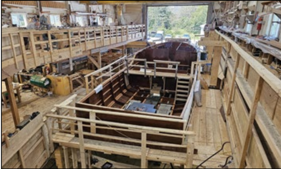
An updated photograph of the Wheeler 55 under construction at Brooklin Boat Yard in Brooklin. They are now beginning to work on her interior and systems.
