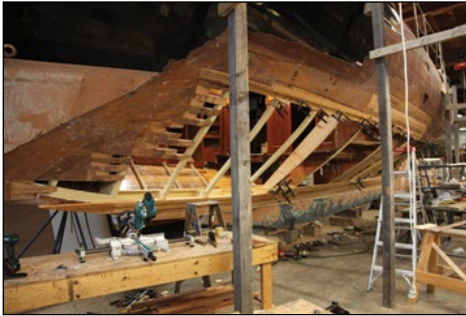
This L. Francis Herreshoff cold moulded hull grounded in Rhode Island last fall. She pounded a number of sizeable holes in her side before being rescued. She was then trucked to Rockport Marine where she is under going extensive repairs. Many of the numerous holes were combined into one big hole as it was much easier to repair.
