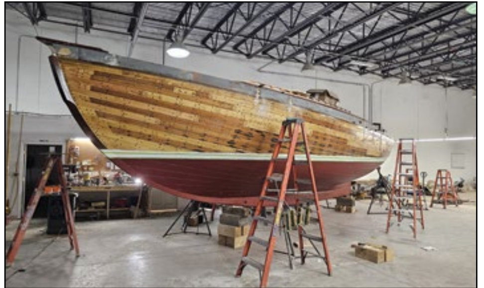
This is an Alden schooner that is being completely rebuilt by Richard Stanley at a facility in Brunswick for her owner.
