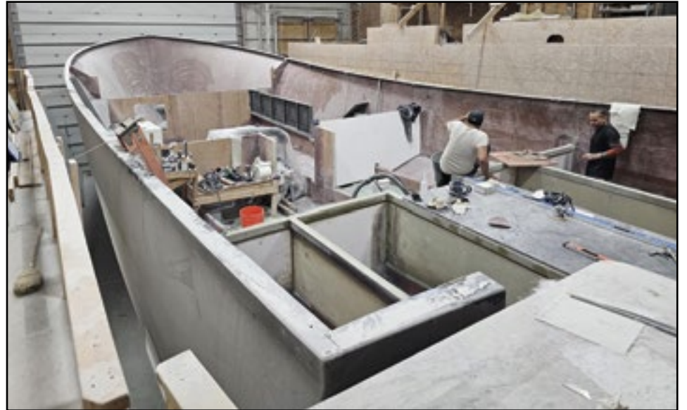
Boricua Custom Boats in Steuben is working on the structure below the platform on this Wesmac 50. Unfortunately, this is as far as they are going as she is up for sale.
