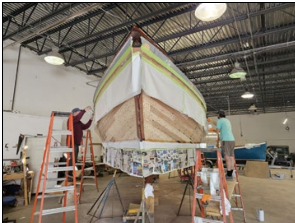
Richard Stanley and Sawyer Theriault working on an Alden schooner in Brunswick. They have finished the hull repairs and was now repairing the bulwarks.
