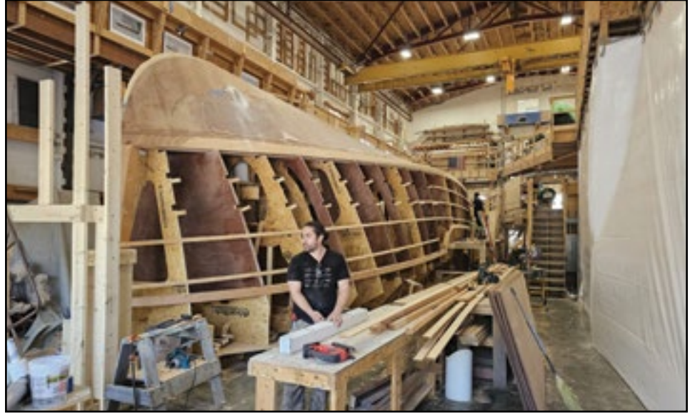
At Brooklin Boat Yard in Brooklin they are building the hull for a 55-foot Wheeler. They have one more of these to do.
