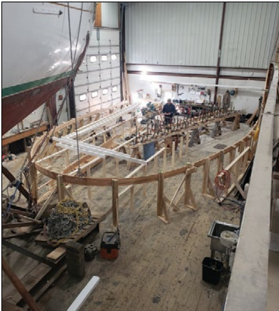
At the Shipyard at Boothbay Harbor, Bristol Marine they are making the frame work for replacing the stern section of the main deck on KATAHDIN, owned by Moosehead Marine Museum of Greenville. When it warms a little bit more they will load this on a truck and head to Greenville to install and have completed before their season begins in June.
