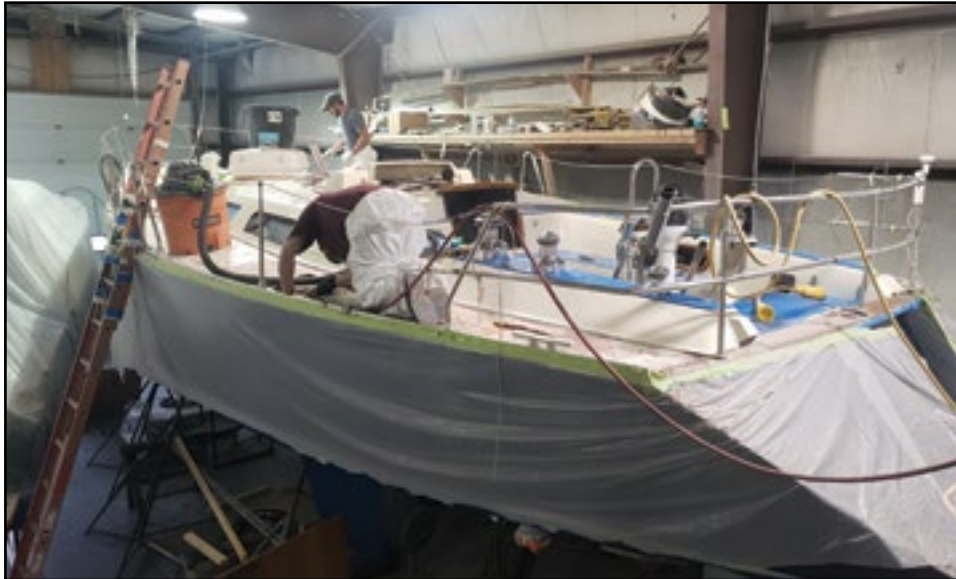
At Johanson Boat in West Rockport they are replacing the core in the deck of this sailboat.
